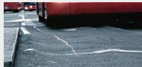
Road surface deformation
